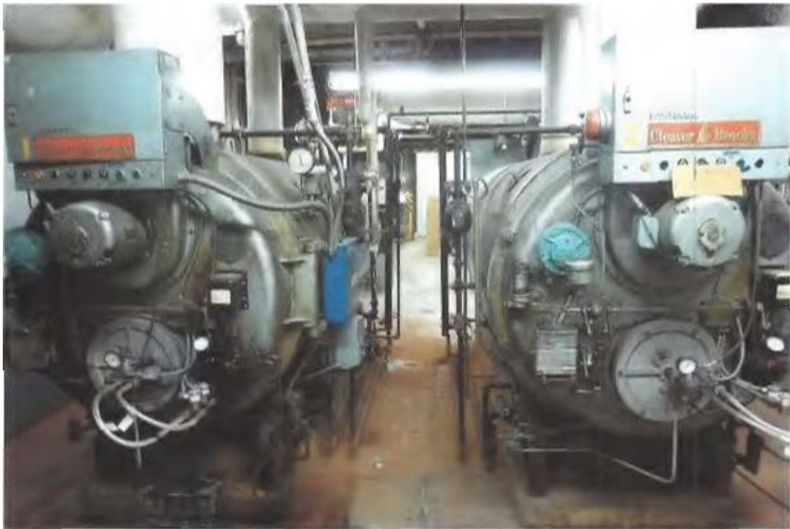
Subject Property — Boilers
